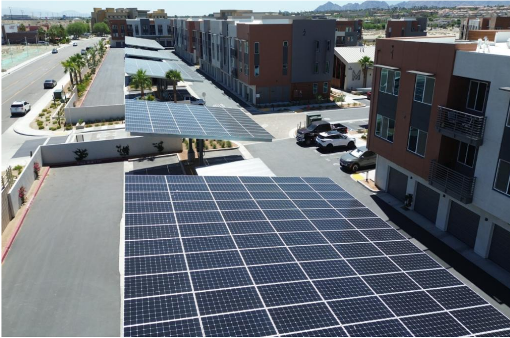
Creates A Megawatt of Power From Carport Roofs
