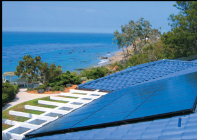
SunPower solar panels used in a 12 kilowatt rooftop system, California
