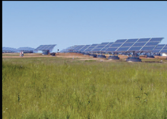
SunPower solar cells used in a 12,000 kilowatt solar power plant, Germany
