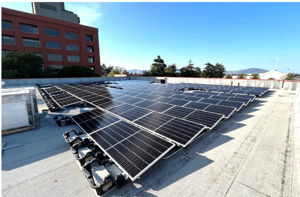
Waterfront Plaza solar system.
